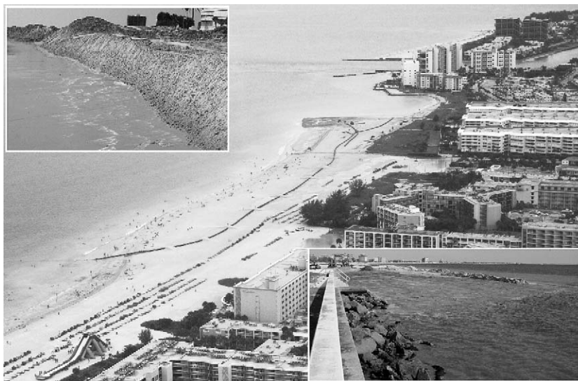
Fig. 5. Construction of the Upham Beach nourishment project. The aerial photo was taken on July 28, 2004, looking north. Inserts: longitudinal dikes near the outflow to control turbidity.
